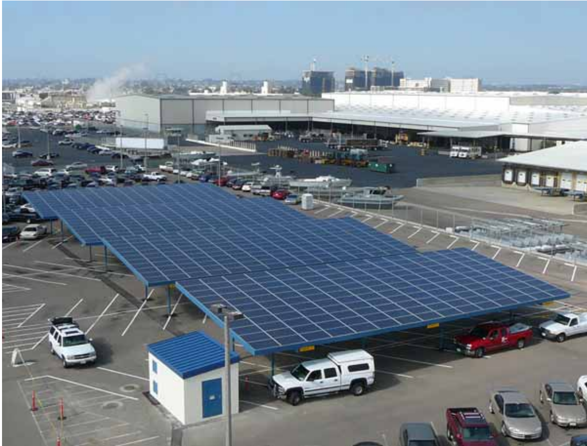
137kW Solar Carport – US Navy
