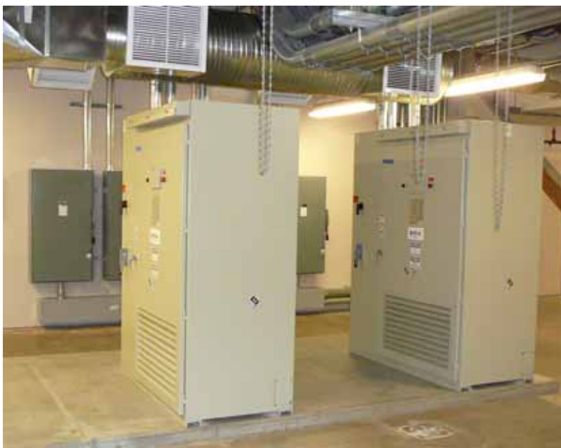
240kWac PV System, Pfizer, San Diego, CA
